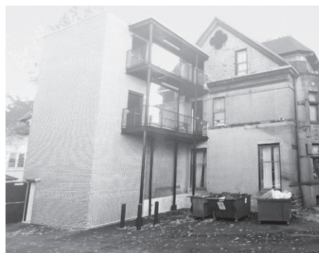
The new stair tower on the north side of the Chapter House.
